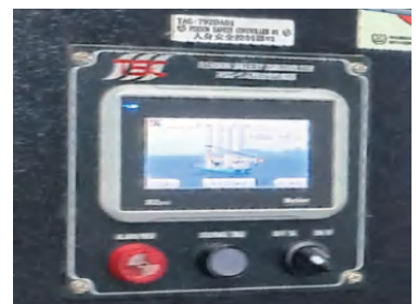
(Extended alarm Panel)
