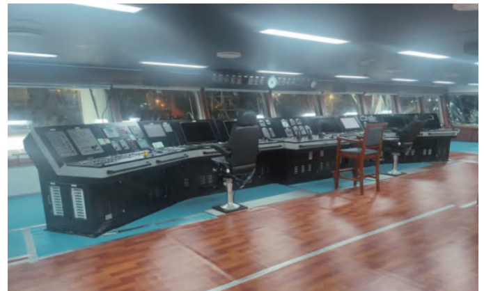
(Wheelhouse Control Console-Front)
