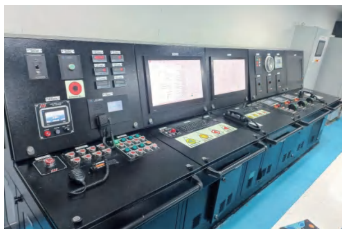
(Engine Room Control Console)
