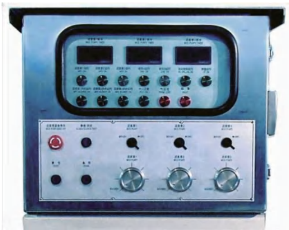
(Local Console of Mud Pump)
