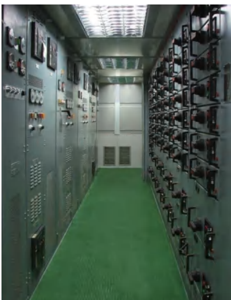
(Electric Control Room-DC)
