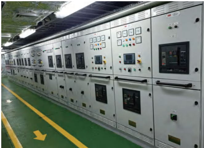
(Gen Control Panel)
