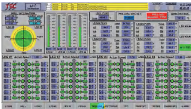
(Jacking System HMI-VFD)
