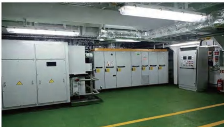
(Main Thrusters VFD and Control Cabinet)
