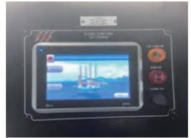
(Personnel Safety System Panel)
