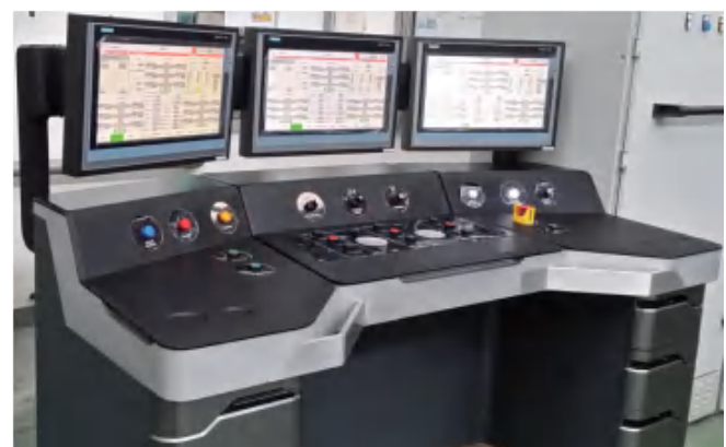
(Central Control Console)
